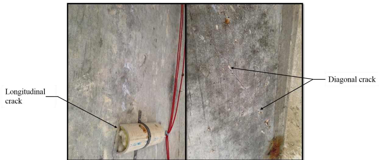
Figure 111. Typical longitudinal and diagonal cracks at the bottom of deck
