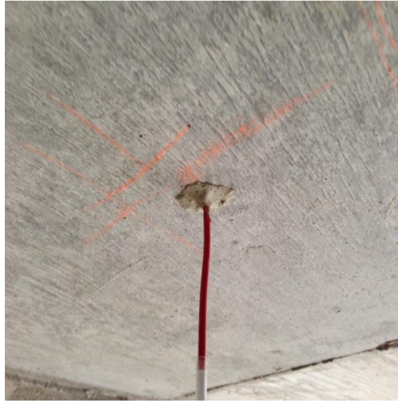
Figure 21. Thermistors at the bottom of deck
